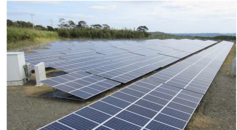
Figure 1 Photovoltaic system in island
